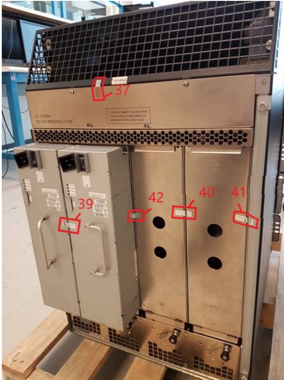
Figure 36 - SRX5800 Tamper-Evident Seal Locations (Rear, Six (6) Seals: TEL 37,39,40-42)
