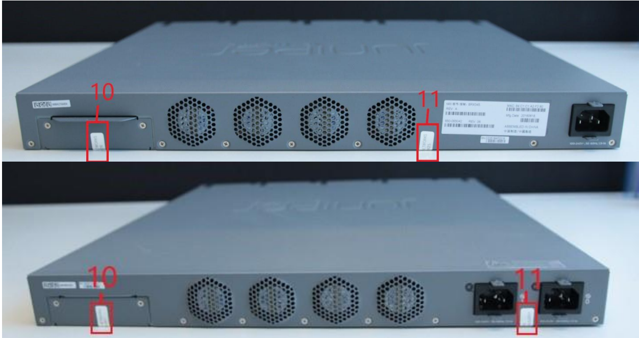
Figure 23 - SRX 340/345 Tamper-Evident Seal Placement (Rear Panel, Two (2) Seals: TEL 10 & 11)
